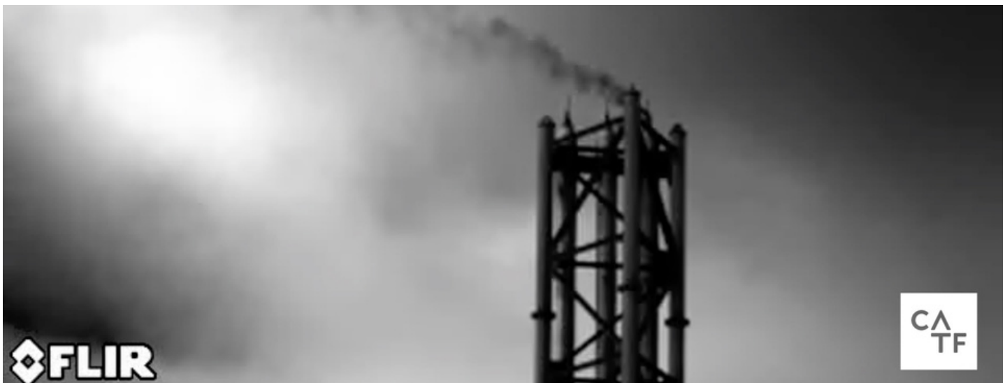
Image: "Broken Emergency Vent Pipe", Clean Air Task Force
